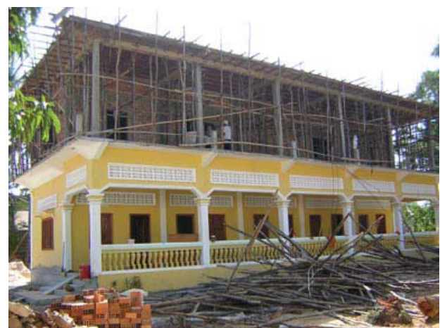
Building the new second story at Wat Chork for a computer lab and language classrooms.
